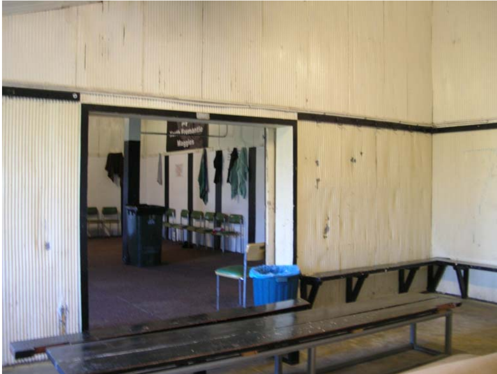
Figure 61 Interior view of the original change rooms. The original lining on the northern wall of this change room has been replaced with new 'Zincalume Custom Orb' wall lining. Hocking Planning and Architecture, August 2009.
