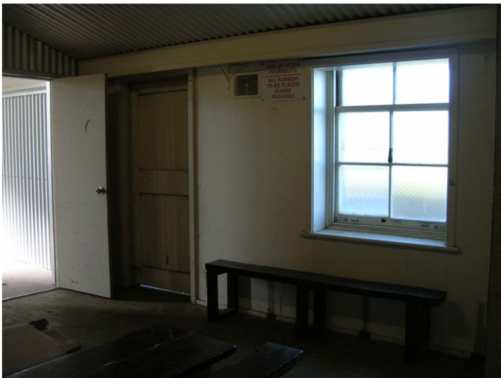
Figure 62 East wall (facing the oval) of the central change room. note lined and raked ceiling, cutting off the head of an existing double hung sash window. It is possible that the ceilings in the change rooms were unlined originally and the full height of the window was accommodated. Hocking Planning and Architecture, August 2009.
