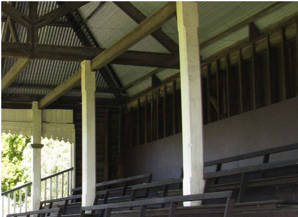
Figure 56 Detail of plywood lining (after conservation work) painted to match the rest of timber structure. Hocking Planning and Architecture, October 2009.
