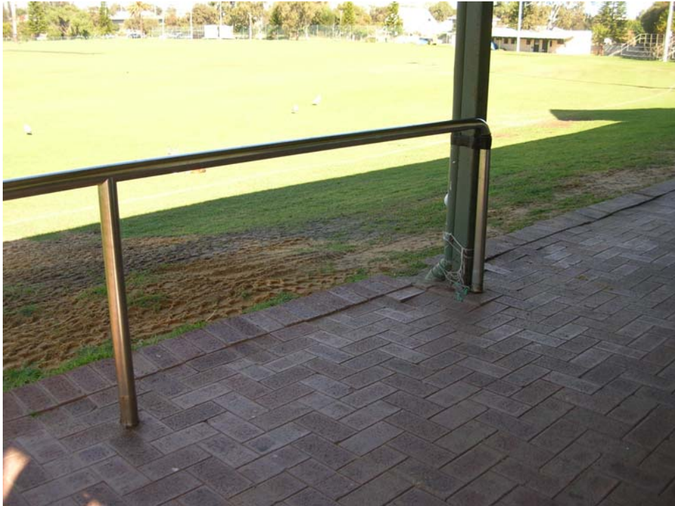
Figure 76 Existing handrail on the eastern bay of the verandah poses a safety risk as the handrail is not secured to the ground. Hocking Planning and Architecture, August 2009.
