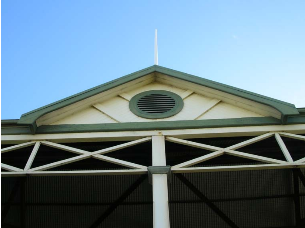
Figure 52 Detail of gable end on the east elevation. Hocking Planning and Architecture, August 2009.
