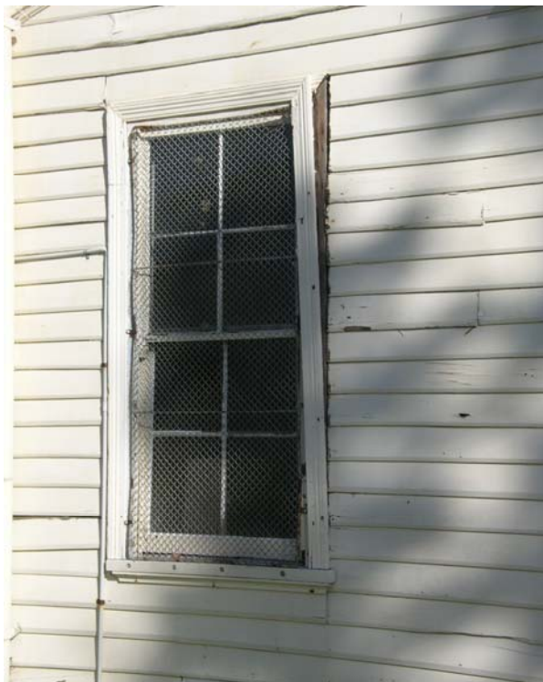
Figure 58 Detail of double hung sash window on the north elevation. Similar maintenance issues and damage to the window architraves and weatherboards are typically observed around the grandstand. Hocking Planning and Architecture, August 2009.
