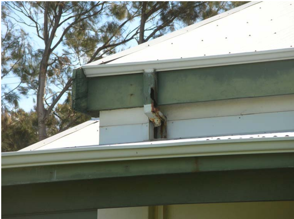
Figure 75 Detail of rusted gutter and downpipe on the main roof. Hocking Planning and Architecture, August 2009.
