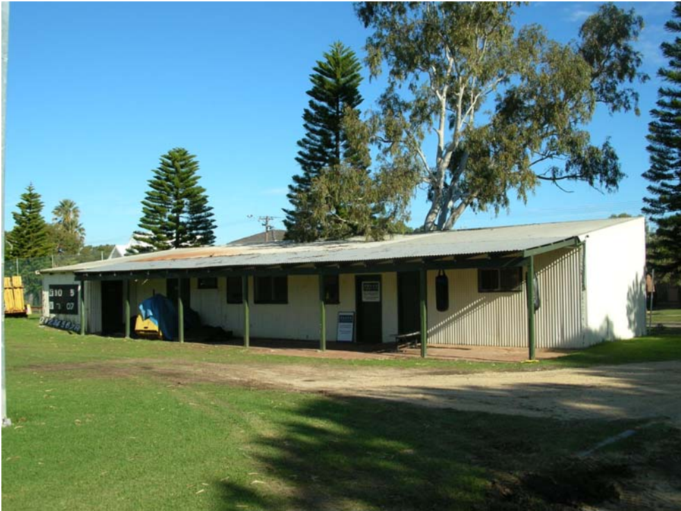
Figure 85 View of former stable from the oval. Hocking Planning and Architecture, August 2009
