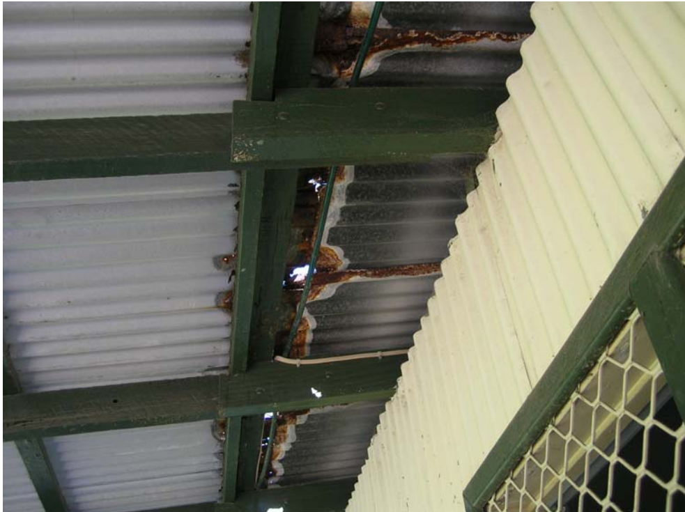
Figure 89 Detail of heavily rusted corrugated sheet metal roof above the verandah. Hocking Planning and Architecture, August 2009
