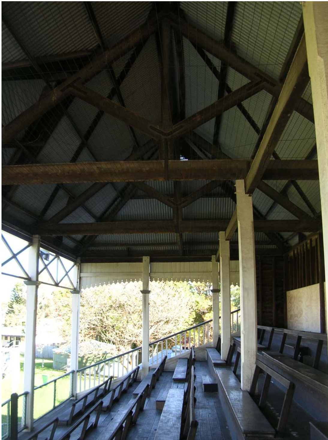
Figure 54 View of the pavilion. The timber roof, columns and wall structures are in relatively good condition and wearing well. Plywood lining (unpainted) on the internal face of the west wall was put in place during a recent repair and conservation campaign. The lining was subsequently painted to match existing timber structure. Hocking Planning and Architecture, August 2009.
