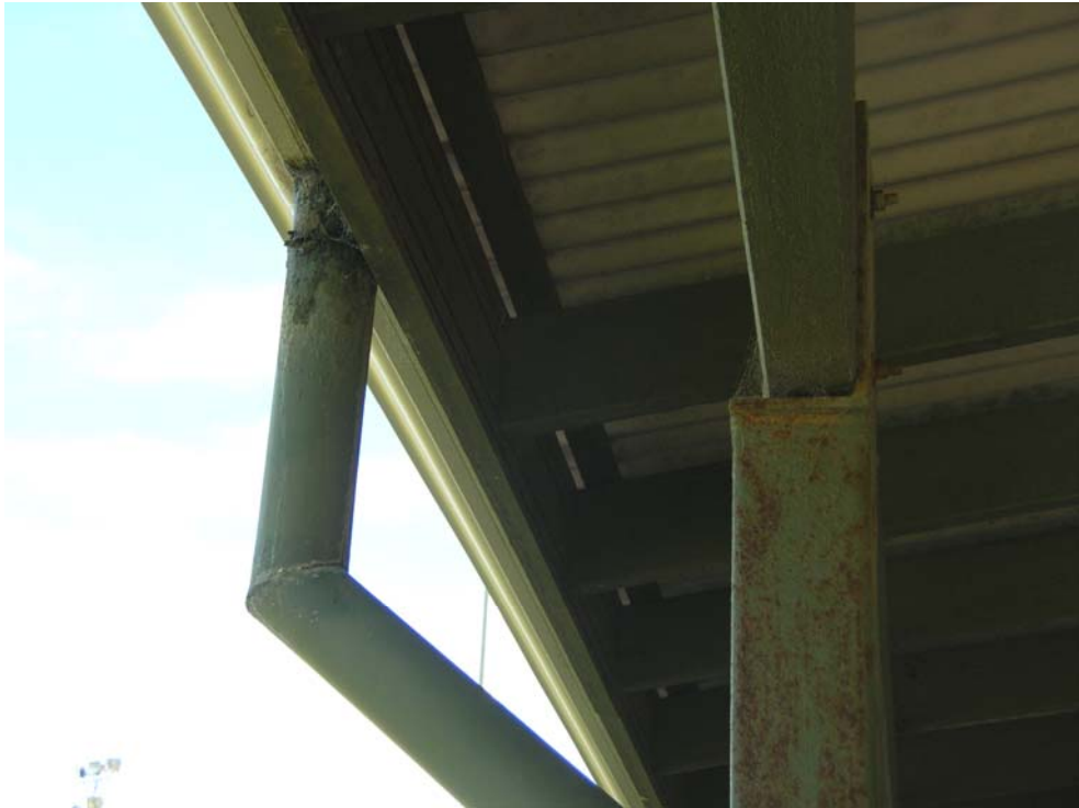
Figure 74 Detail of rusted gutter and downpipe along roof above verandah. Hocking Planning and Architecture, August 2009.
