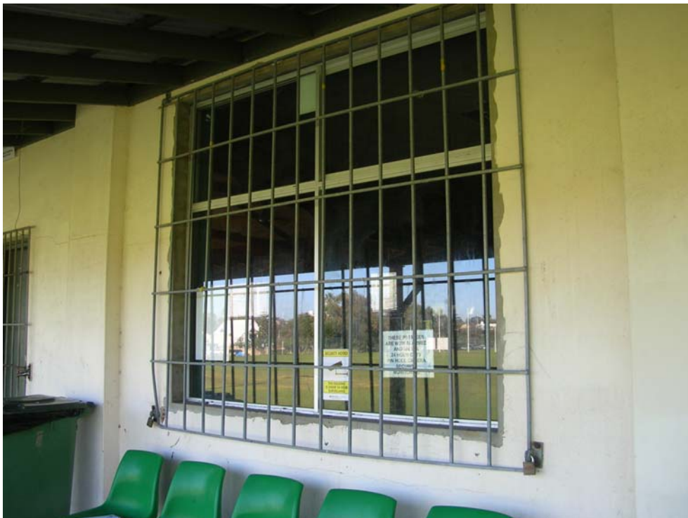
Figure 73 Detail of existing window on the south elevation. Hocking Planning and Architecture, August 2009.
