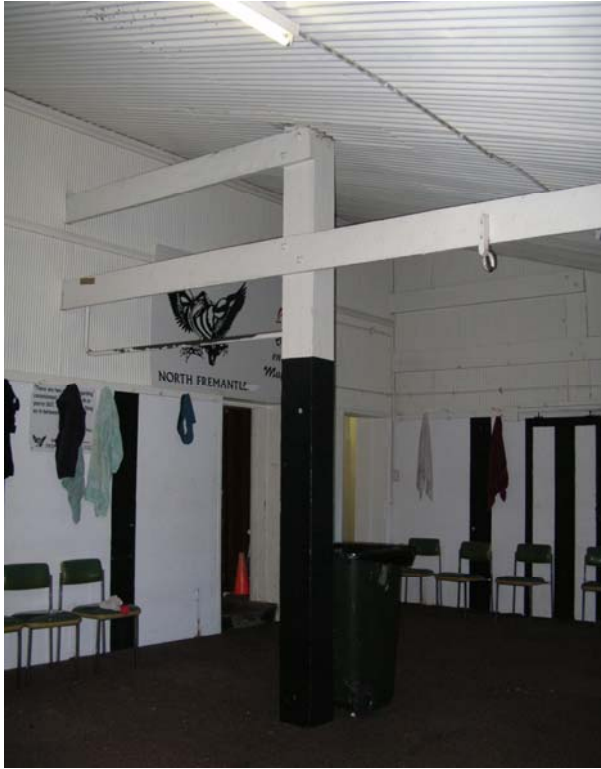
Figure 59 Interior view of the original change rooms below the pavilion. The structural columns carry through to support the roof structure above. Hocking Planning and Architecture, August 2009.
