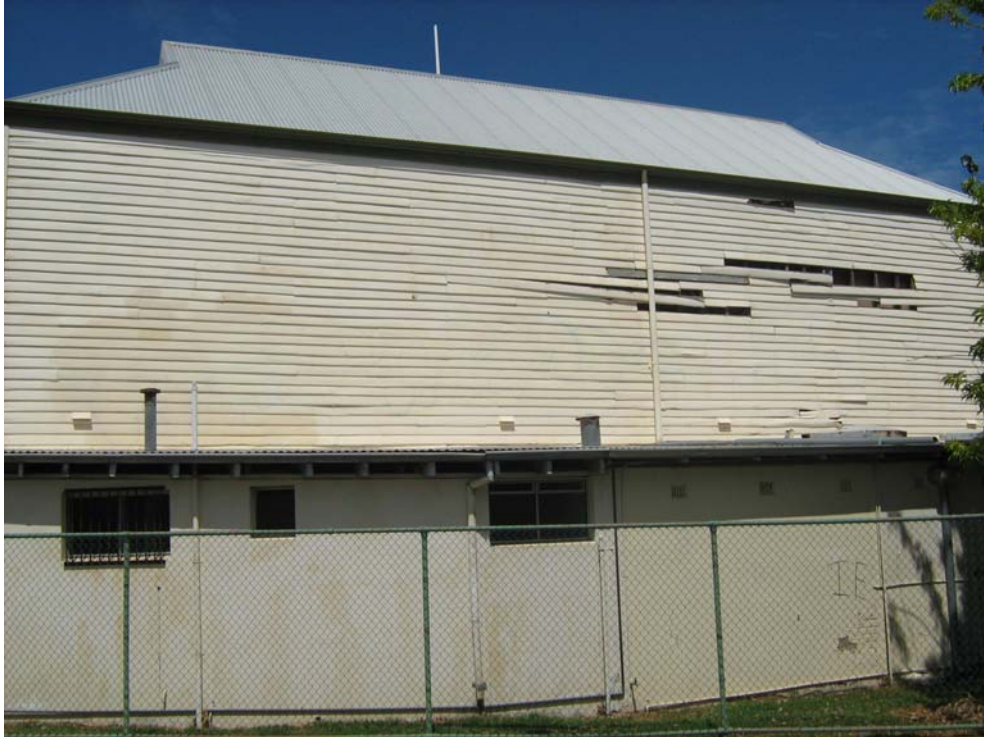
Figure 48 View of the grandstand (north elevation) prior to conservation work. At the time of inspection, the process of removing sections of termite affected jarrah weatherboard and structural timber were in progress. Hocking Planning and Architecture, August 2009.
