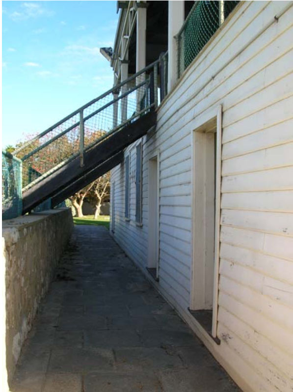
Figure 50 View of the ground floor level of the grandstand, sunken and concealed behind a limestone retaining wall as the ground level of the oval and surrounding grassed area were elevated over the years. Hocking Planning and Architecture, August 2009.
