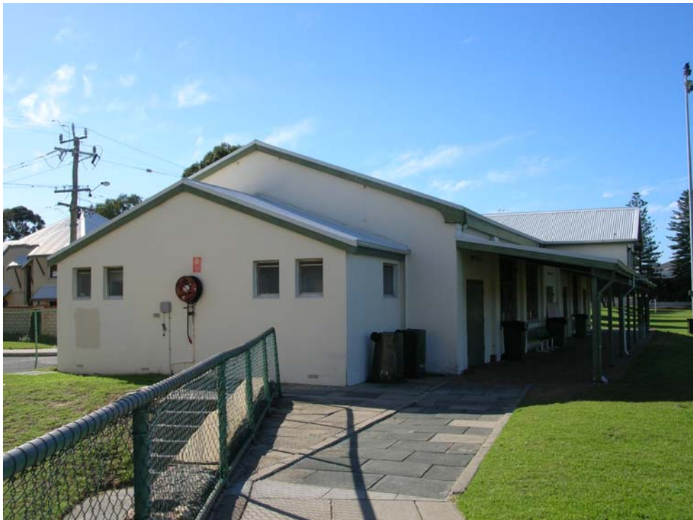
Figure 69 View of toilet annexe, west elevation of the hall. Hocking Planning and Architecture, August 2009.
