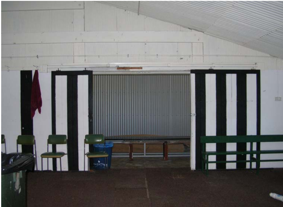
Figure 60 View of the central change room from the southern end change room. The original interiors including, sliding doors between rooms, wall lining and benches re largely intact. However, at the time of inspection, the traditional 'Ripple' corrugated sheet metal lining are being removed and replaced with 'Zincalume Custom Orb' which has larger corrugation profiles. This altered the proportion and general appearance of the original interiors significantly. Hocking Planning and Architecture, August 2009.
