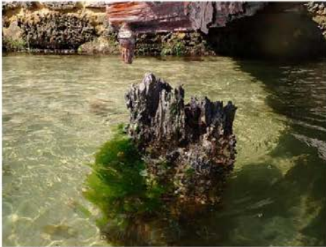
Pile 1A Failure
