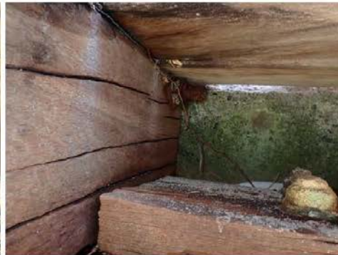
Stress cracking internal face (1)
