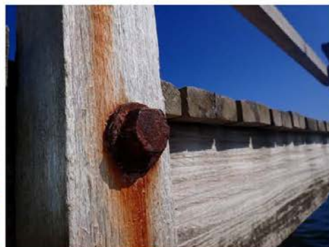
Handrail fixing condition (1)
