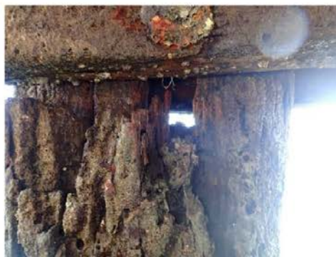
Pile 2B severe splitting and rotting
