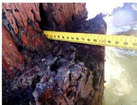
Pile 1B severe wood rot
