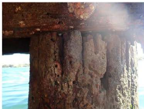
Pile 2A poor condition
