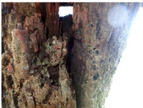
Pile 2B poor condition
