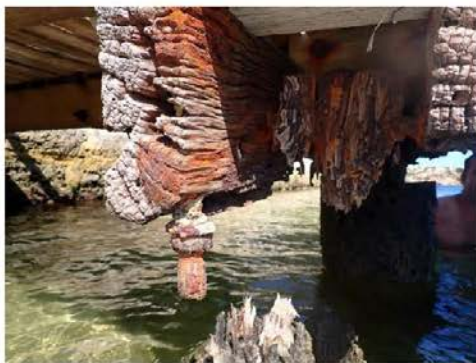
Bent one headstock condition
