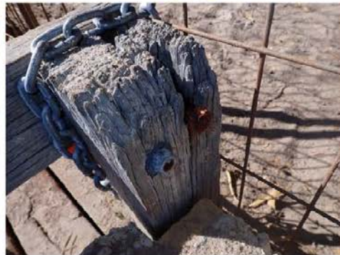
Handrail Timber splitting (2)
