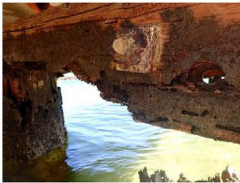
Bent one headstock condition (1)
