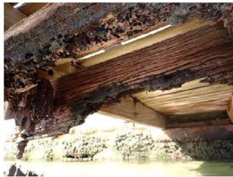
Bent one headstock condition (2)
