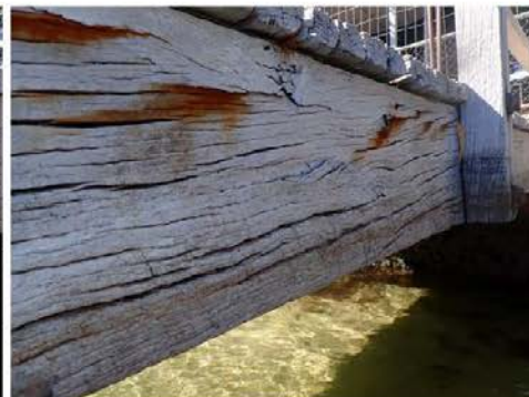
Stress cracking external face
