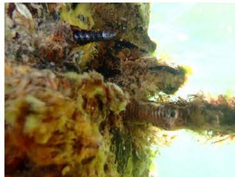
Jetty Ladder exposed coach bolts
