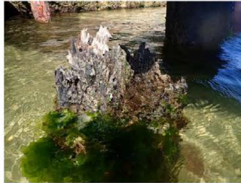
Pile 1A Failure (1)
