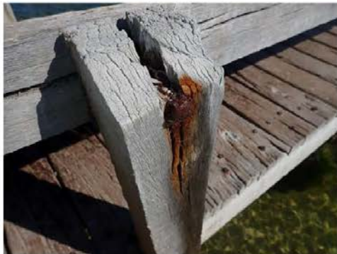
Handrail Timber splitting (1)
