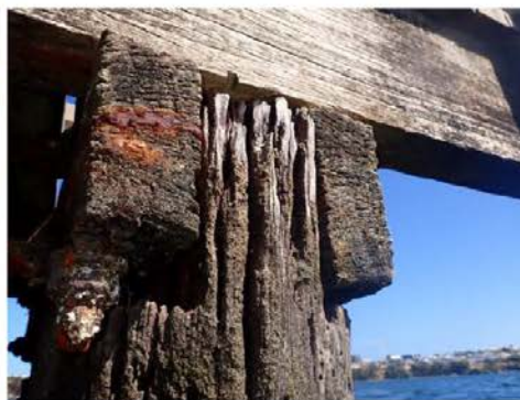
Pile 2A severe splitting
