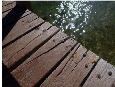
Fixings proud of decking
