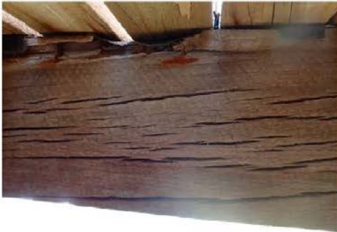
Stress cracking internal face
