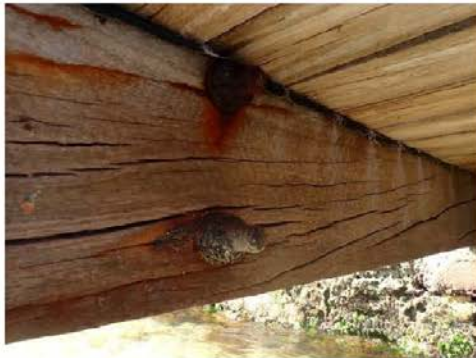
Stress cracking internal face
