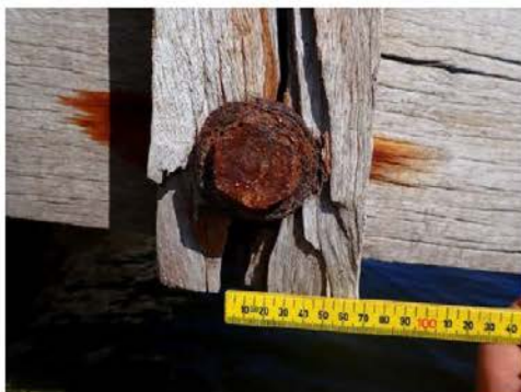
Handrail fixing condition
