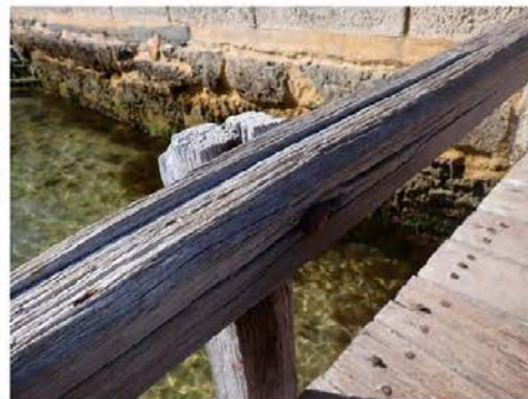
Handrail Timber splitting
