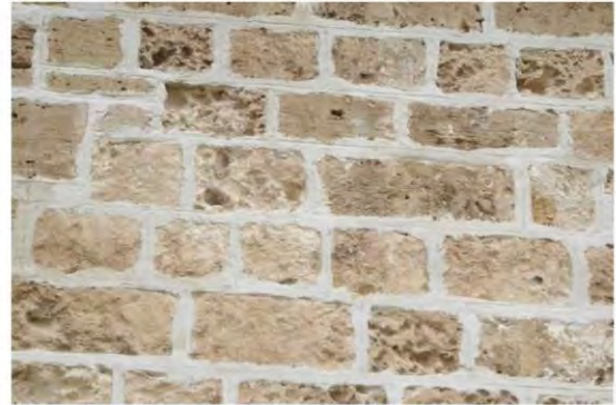
Figure 91: Typical stonework with pointing form 2004
