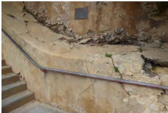
Figure 1: Failing render to steps from High Street
