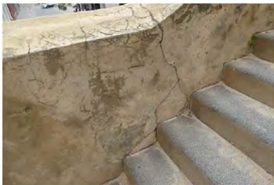
Figure 3: Failing render to steps from High Street
