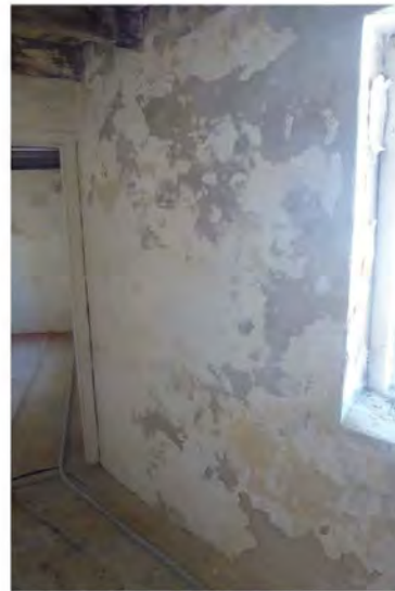
Figure 162: Failing paint and render to west wall Room 14
