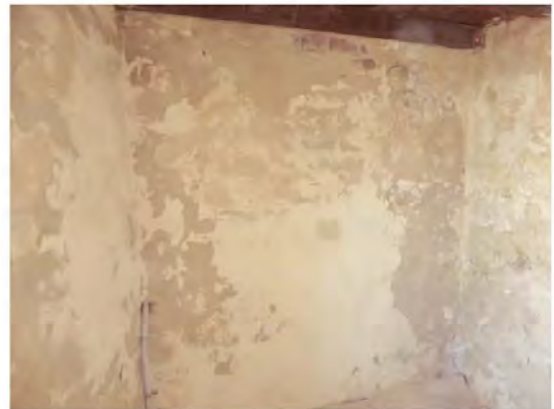
Figure 164: Failing paint and render to west wall Room 13
