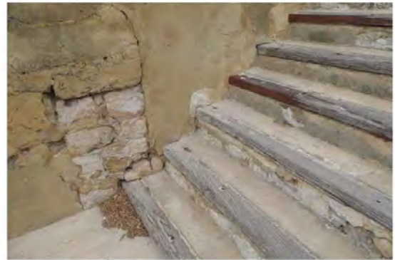
Figure 10: Timber nosings to steps to Round House
