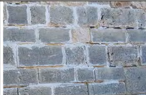
1975 cement (?), (behind 2004 eroded)
