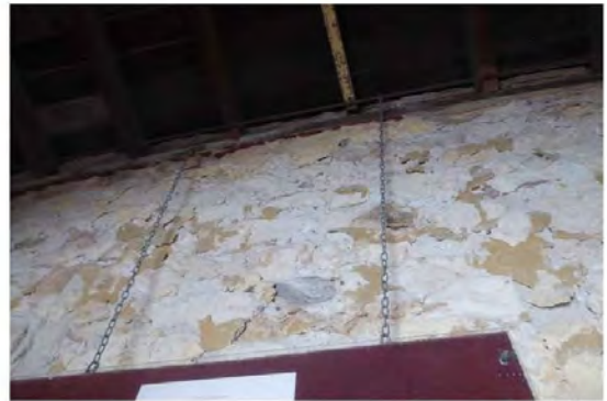
Figure 176: Wearing paint finish to cells
