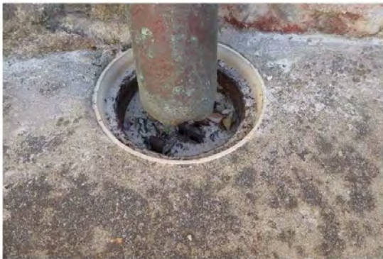
Figure 105: Silted up drain
