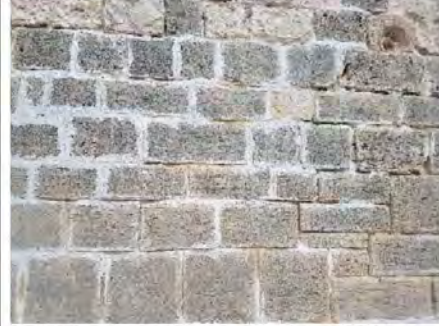
2004 lime mortar – weathered and friable
