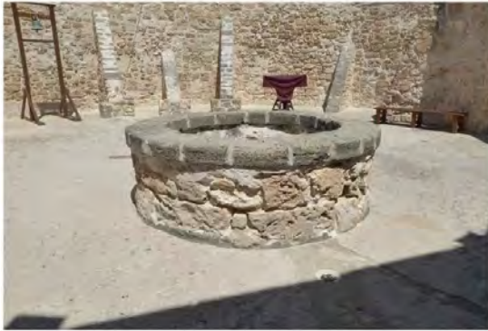
Figure 131: Eroding joints to well
