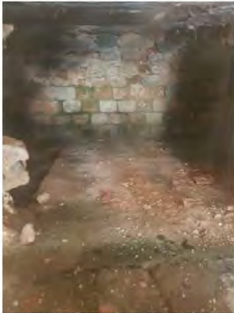
Figure 57: Evidence of recent fretting of bricks in oven roof
