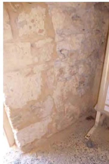
Figure 178: Previous repairs to limestone
