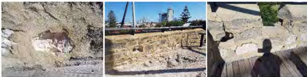
Figure 66: Weathered limestone walls
