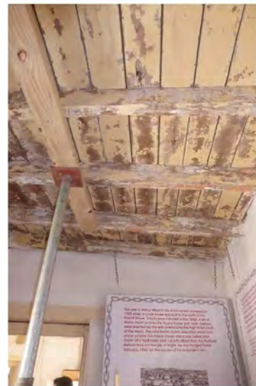
Figure 146: Failing paint to ceiling in Room 2
