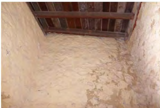
Figure 177: Wearing paint finish to cells
