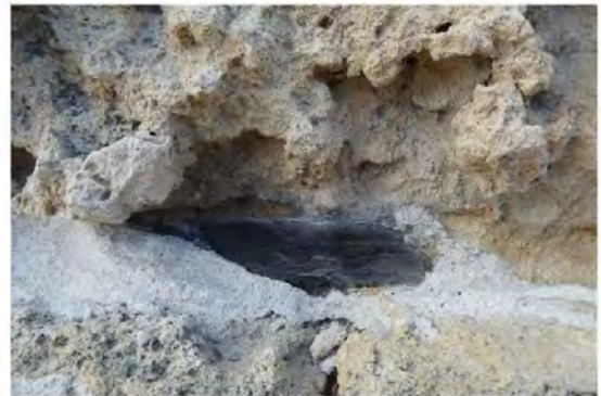
Figure 62: Eroded joint revealing packer
