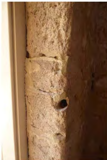
Figure 183: Eroding mortar and stones
