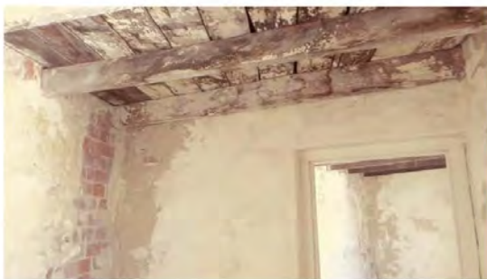
Figure 159: Brick infill and wearing point
