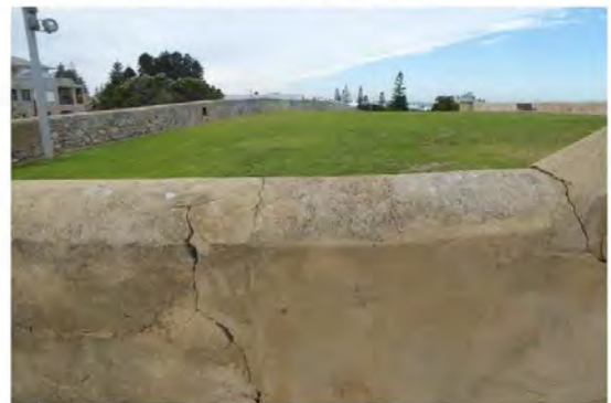
Figure 12: Cracked render to balustrade
