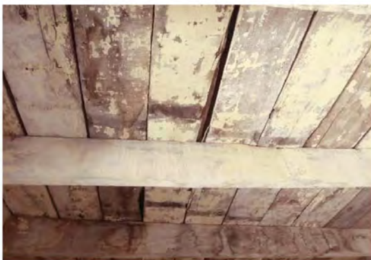
Figure 165: Wearing paint to ceiling in Room 13
