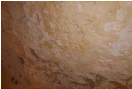
Figure 175: Wearing paint finish to cells
