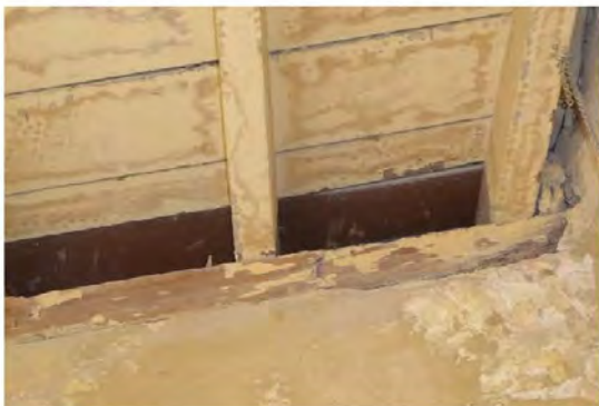
Figure 189: Failing paint to ceiling
