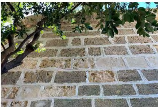
Figure 67: Face 10 repairs and eroding limestone
