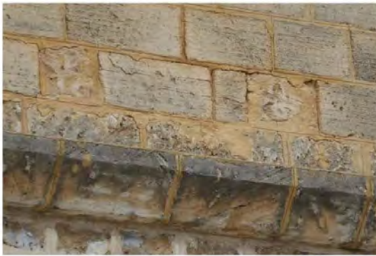
Figure 21: Fretting limestone and missing mortar
