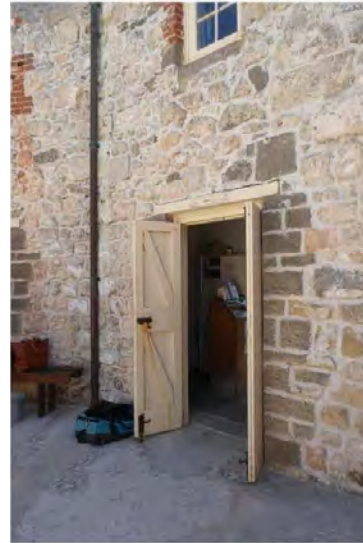
Figure 100: Entry doors with rust staining
