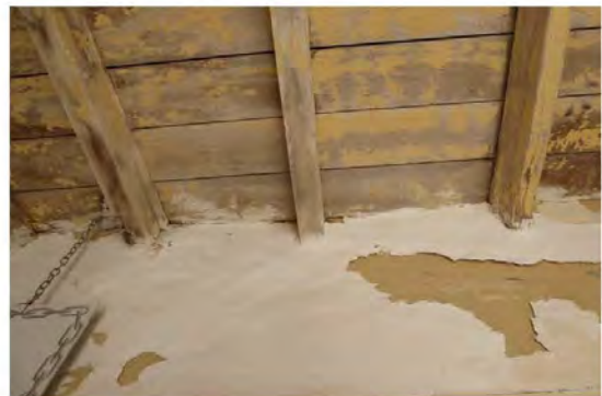
Figure 142: Falling paint due to damp
