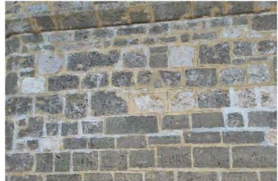
Figure 96: Evidence of previous repairs to external walls
