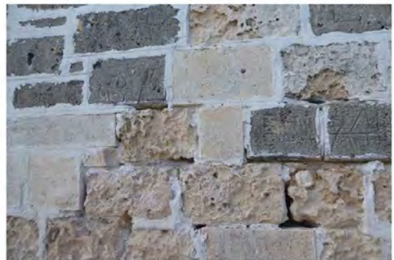
Figure 60: Previous repairs and eroded joints
