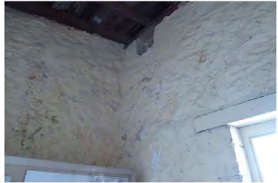
Figure 174: Wearing paint finish to cells
