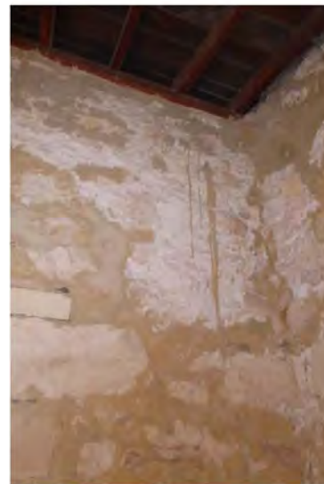
Figure 184: Wearing paint finish to cells
