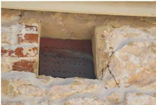
Figure 127: Eroding brick to vent
