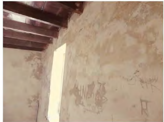
Figure 168: Failing paint and render to west wall Room 15
