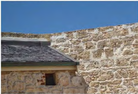
Figure 133: Flashings to roof need inspection
