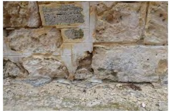
Figure 50: Eroded joints and limestone
