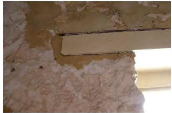
Figure 182: Previous repairs around Intel
