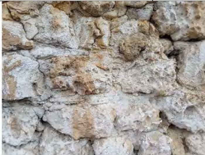
Original mortar (?) with calcium carbonate shell to surface and extensive salt deposits from ground water movement – stair wall
