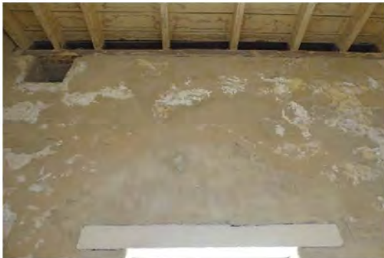
Figure 193: Wearing paint finish to cells
