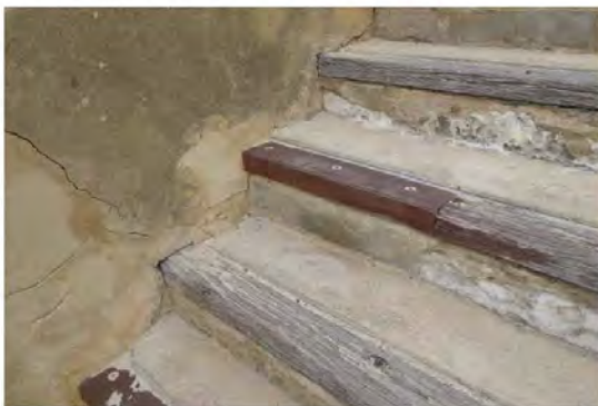
Figure 11: Timber nosings to steps to Round House
