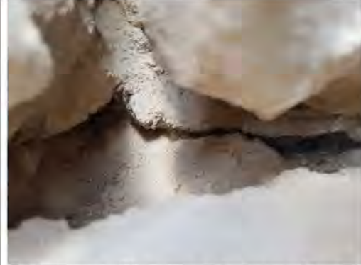
Original mortar (?) appears to have turned back to sand
