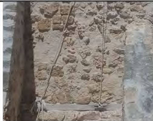
2004 lime mortar – friable mortar build-up beneath original surface of conservation works mortar
