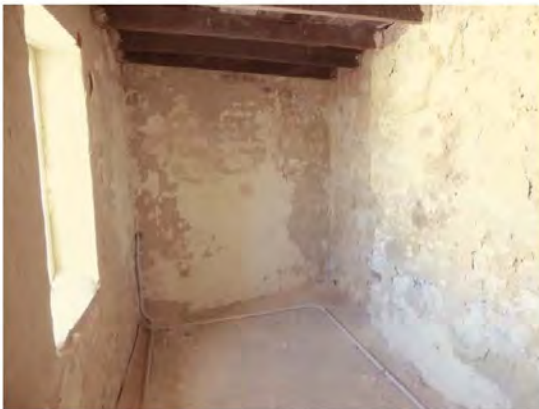
Figure 163: Failing paint and render to west wall Room 13
