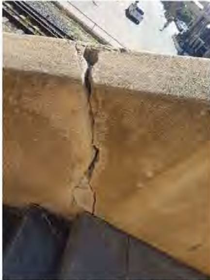
Figure 67: Longstanding, severe, but stable crack to walls of steps
