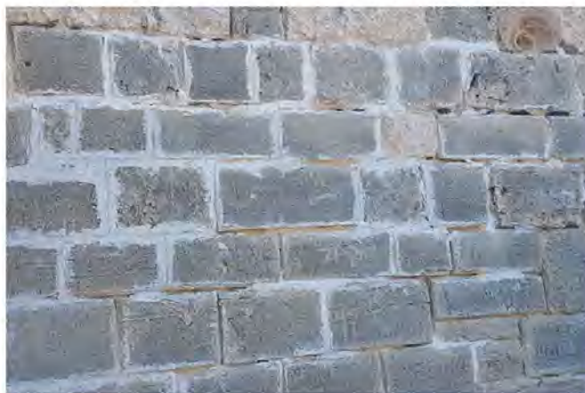
Figure 37: 2004 re-pointing now weathering from joints
