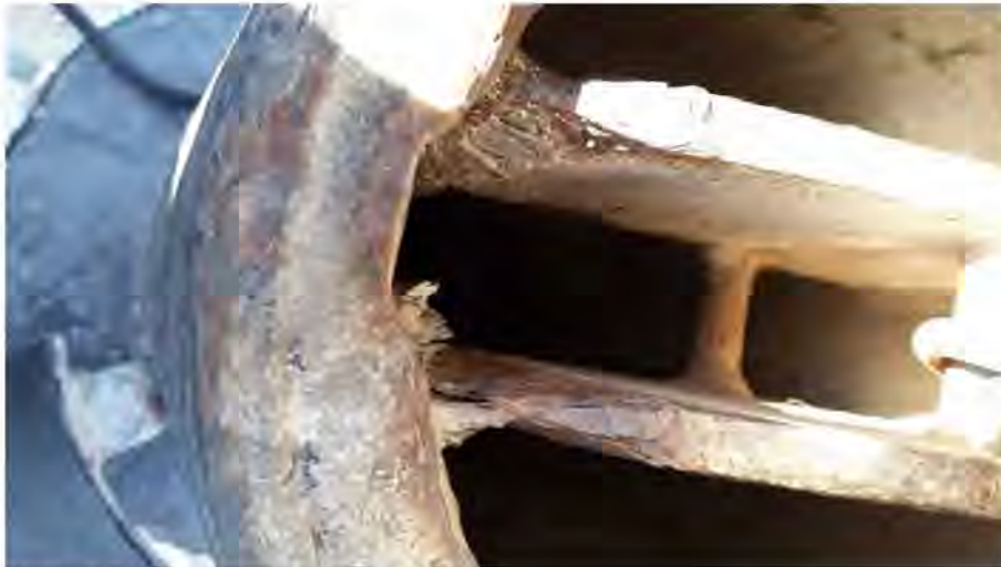
Figure 63: Corroded Pulley plates
