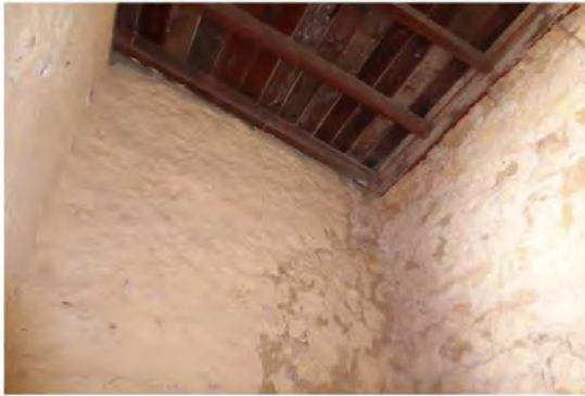
Figure 173: Wearing paint finish to cells
