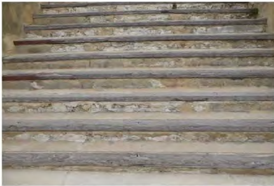
Figure 9: Timber nosings to steps to Round House
