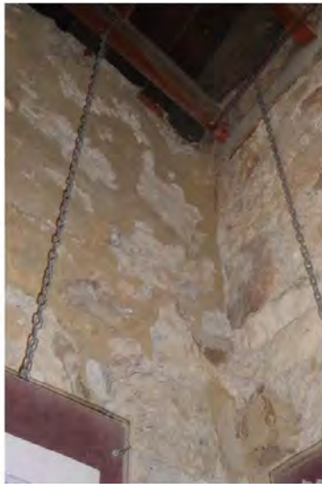
Figure 181: Wearing paint finish to cells
