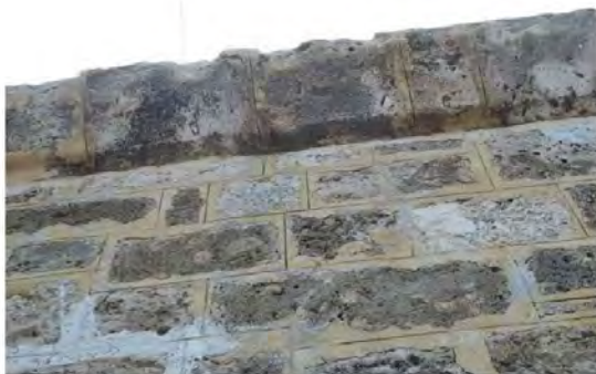
Figure 51: Eroded string course stone
