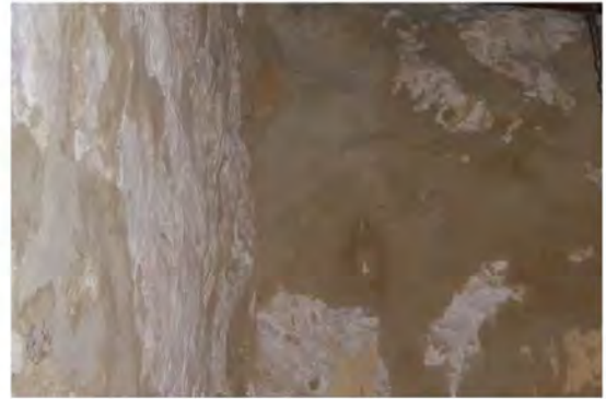
Figure 180: Previous cement repairs
