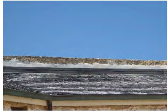
Figure 132: Shingle roof – need closer inspection
