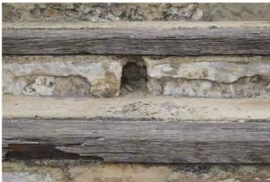
Figure 13: Missing mortar to risers
