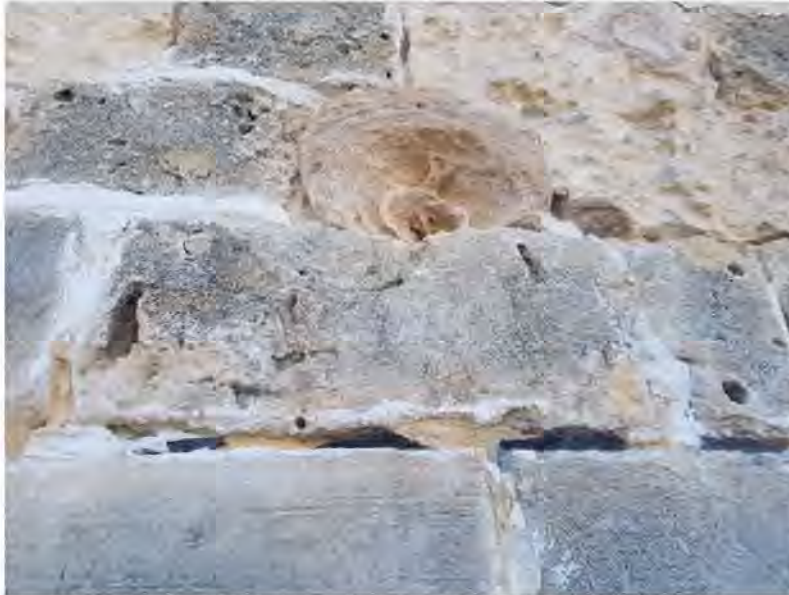
Figure 29: Natural strata of limestone block causing cavity in face
