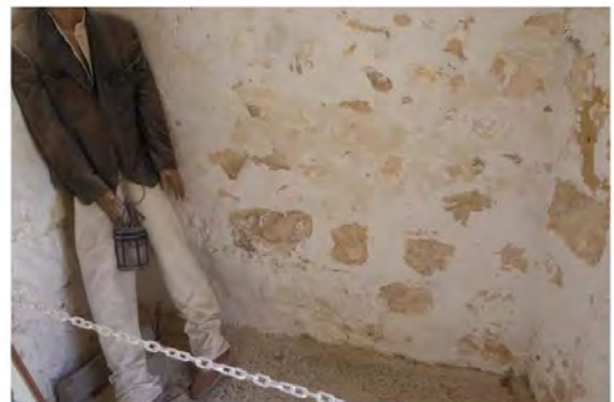
Figure 196: Wearing paint finish to cell 2
