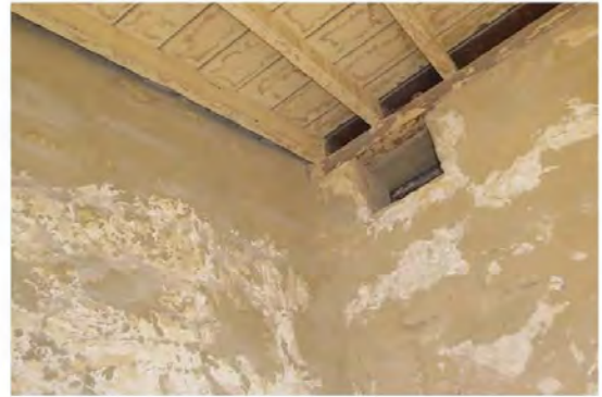
Figure 186: Wearing paint finish to cells
