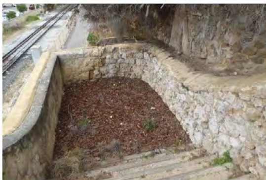
Figure 5: Collected debris in remnant step landing
