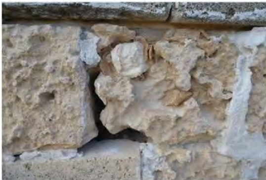
Figure 61: Completely eroded joint
