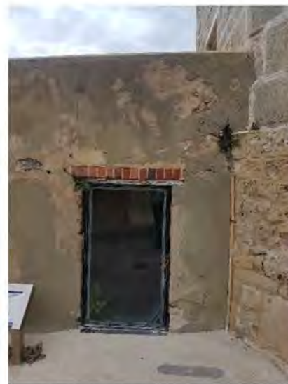
Figure 58: Current sealed door
