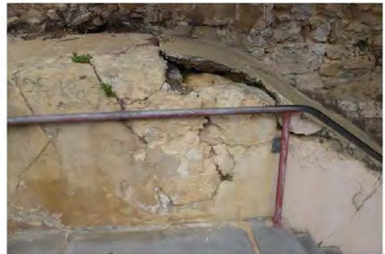
Figure 2: Failing render to steps from High Street
