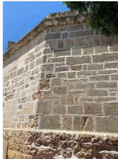
Figure 76: Eroding stone face 11
