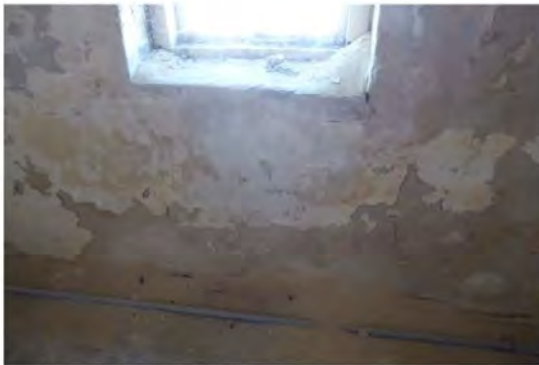
Figure 161: Failing paint and render to west wall Room 14
