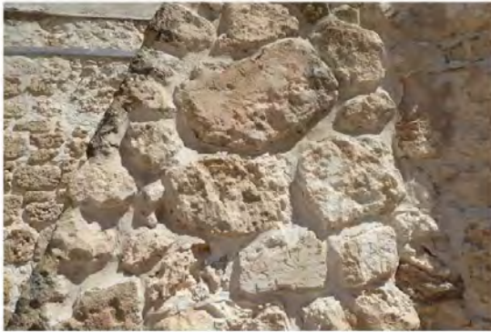
Figure 113: Eroding joints to 2004 mortar repairs
