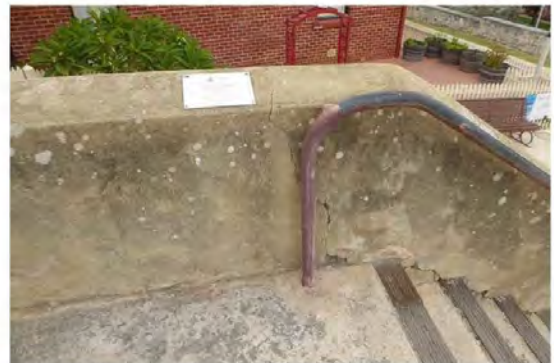
Figure 14: Cracked render to balustrade
