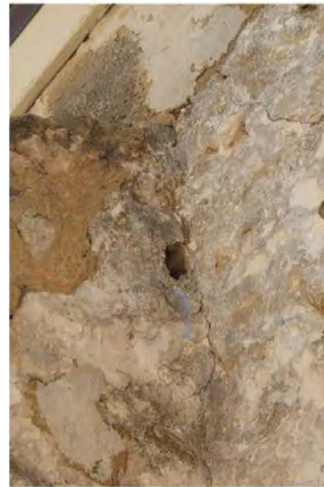
Figure 126: Erosion of stones
