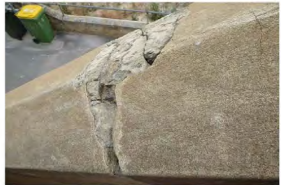
Figure 8: Failing render to steps from High Street
