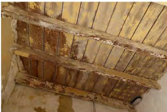
Figure 141: Wearing paint to ceiling
