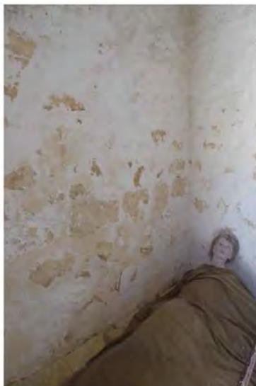
Figure 195: Wearing paint finish to cell 2
