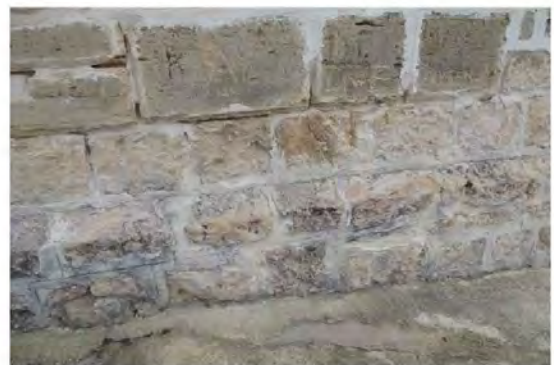
Figure 40: Eroded and repaired joints
