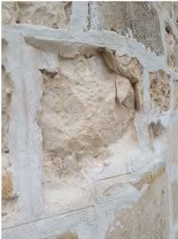
Figure 28: Limestone block weathering NE external wall
