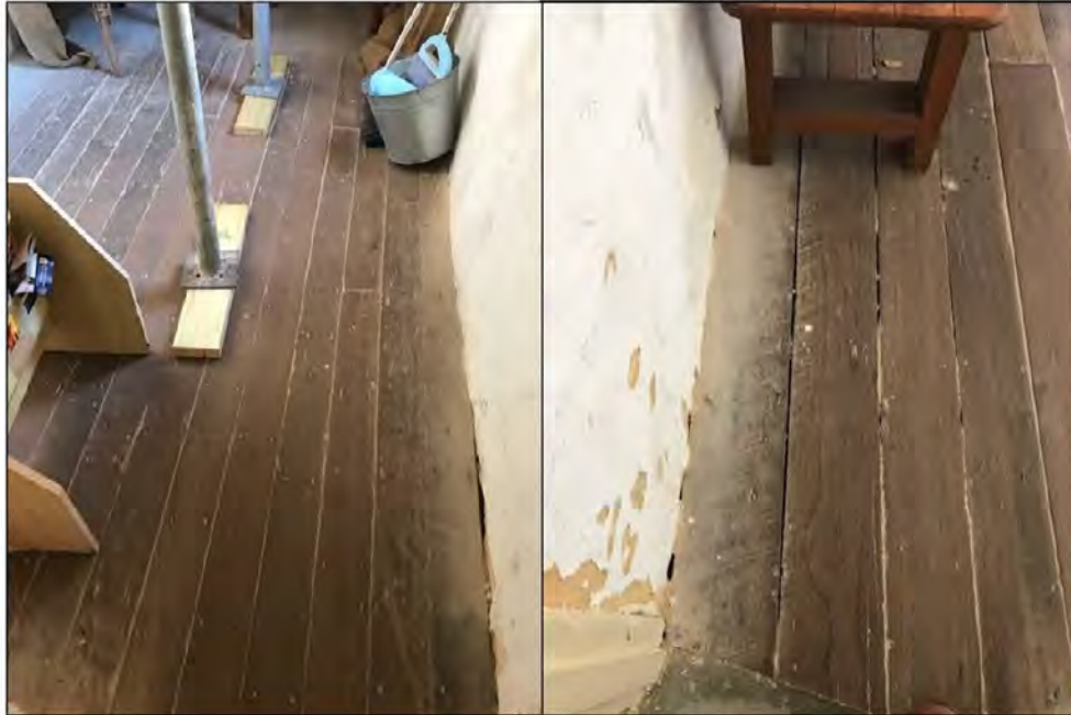
Plate 17. Timber flooring at entrance of the Round House (note gaps between boards)
