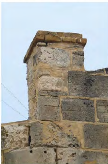
Figure 19: Missing mortar to parapet elements
