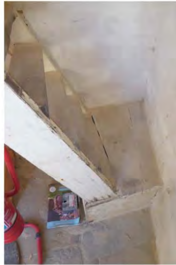
Figure 158: Tight bottom step of timber stair
