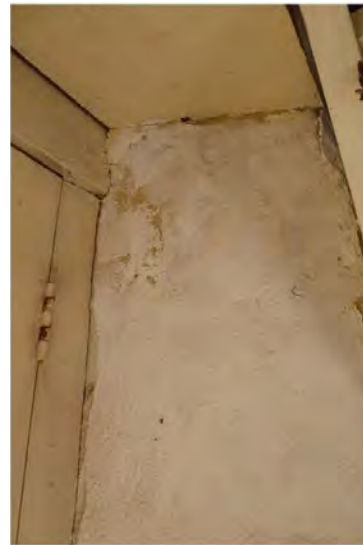
Figure 138: Damaged render caused by damp
