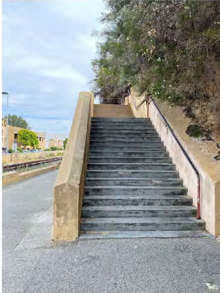
Plate 9. View of northern staircase from street level, gauge railway to left (note modern concrete steps)
