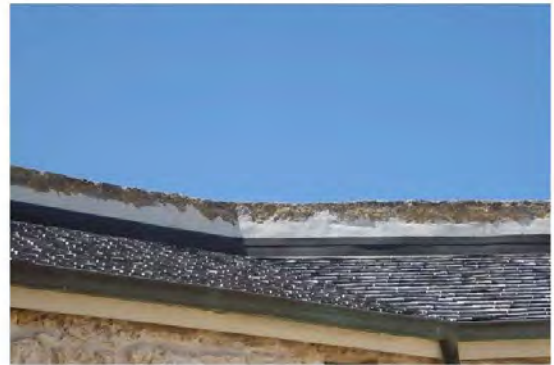
Figure 134: Shingle roof – need closer inspection
