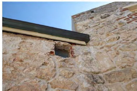
Figure 130: Air vent and replacement gutters
