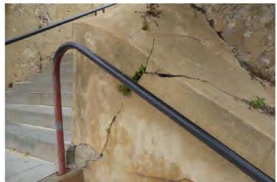
Figure 4: Failing render to steps from High Street
