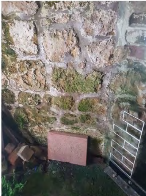
Figure 55: Biological growth on bakehouse walls
