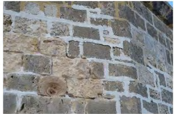
Figure 64: Repairs and eroded limestone
