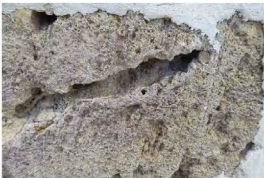
Figure 45: Defects in limestone
