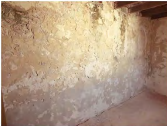
Figure 167: Failing paint and render to west wall Room 15
