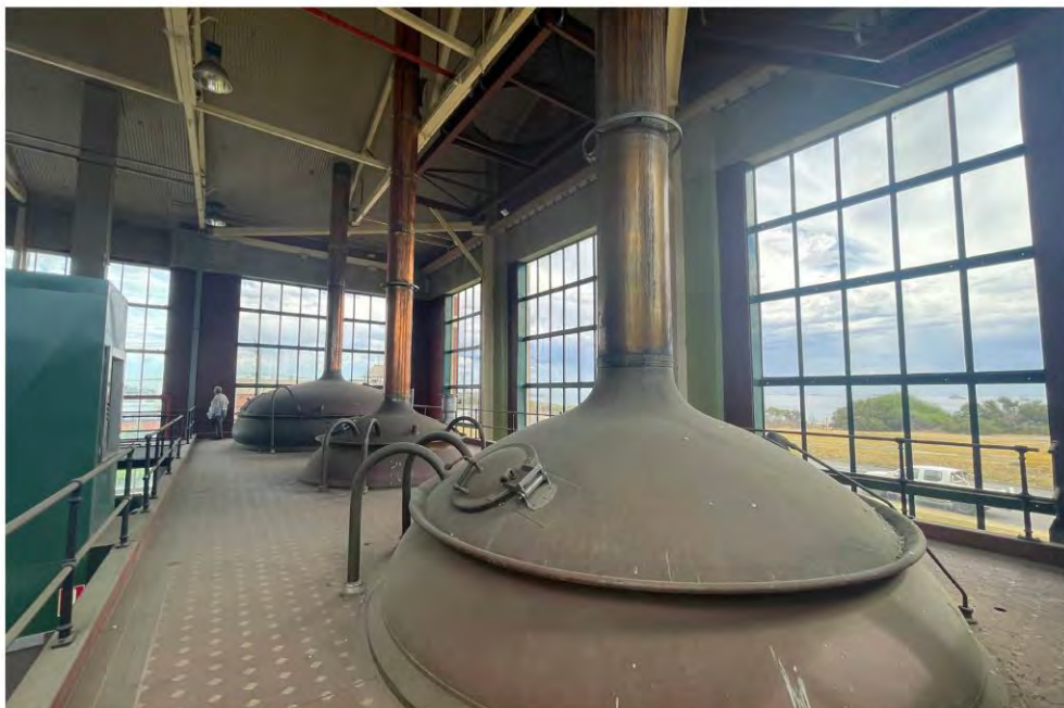
20 Internal - Factory Building: Mezzanine level (Kettles/VATS)
