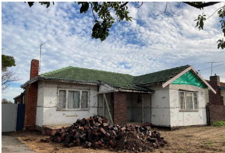
93 Collick Street following the removal of the 1970s brick veneer cladding to reveal the largely intact original Hilton house, June 2021. The brick tie straps were fixed to the face of the original external wall cladding.
