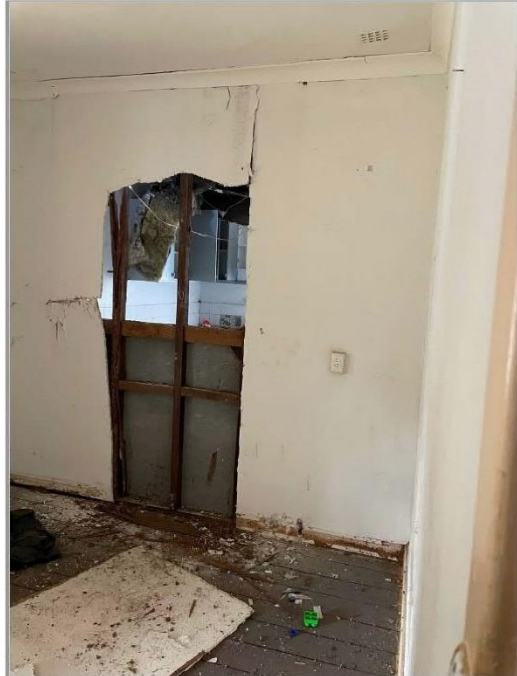
PHOTOGRAPH 11 Bedroom 2. Wall cladding removed to reveal termite damaged timber wall studs and noggings to internal wall of house.
