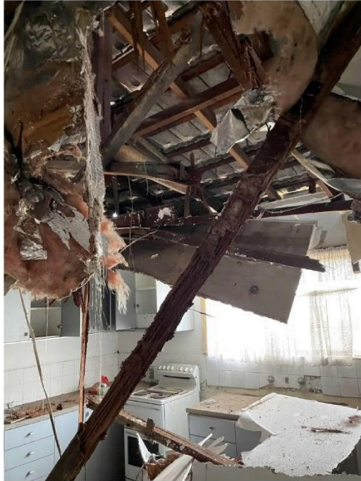
PHOTOGRAPH 13 Kitchen. Collapsing ceiling and termite damaged ceiling joists.
