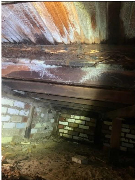
PHOTOGRAPH 14 Sub-floor space (from termite inspection report June 2021). Termite damaged floor joist and extensive white mould fungal wood rot.
