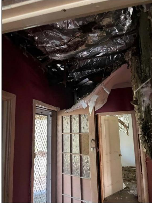
PHOTOGRAPH 9 Interior of Hall showing collapsed ceiling.
