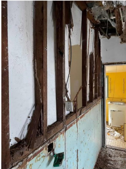
PHOTOGRAPH 12 Kitchen looking toward enclosed rear verandah – other side of wall shown in photograph 10. Termite activity in timber wall studs and collapsing ceilings with termite damaged ceiling joists.
