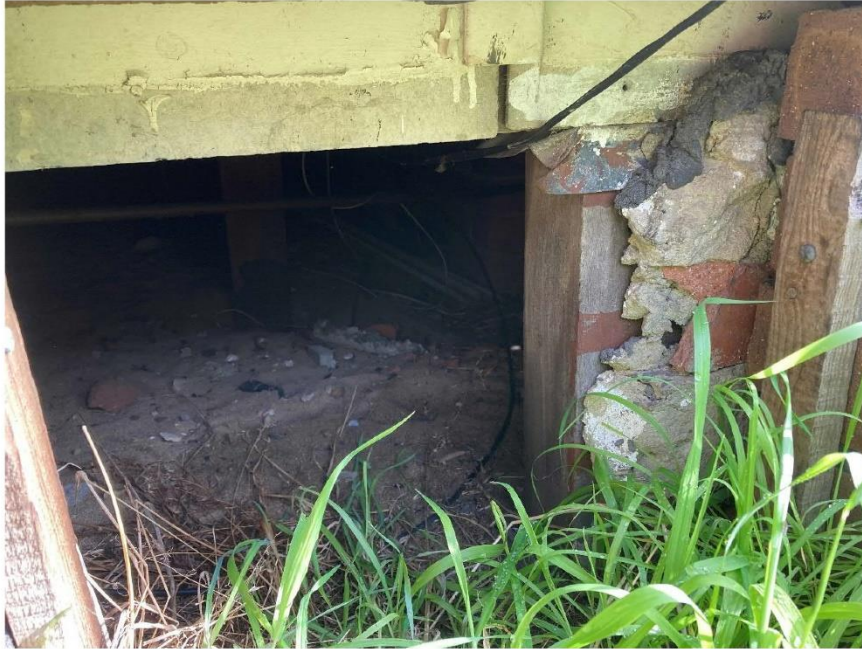
PHOTOGRAPH 7 Sub-floor access hole, east elevation. The original asbestos clad stud framed wall can be seen behind the later brick veneer addition indicating that the original external wall cladding and trims are still intact and were not removed when the veneer was added.
