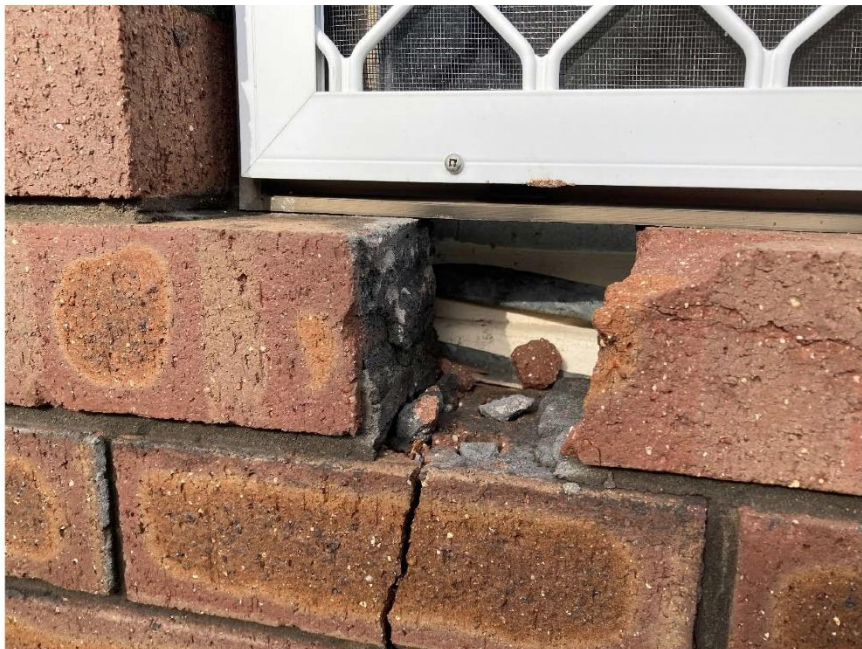
PHOTOGRAPH 8 The original asbestos wall cladding and window sill can be seen where part of the brick veneer cladding has been removed.
