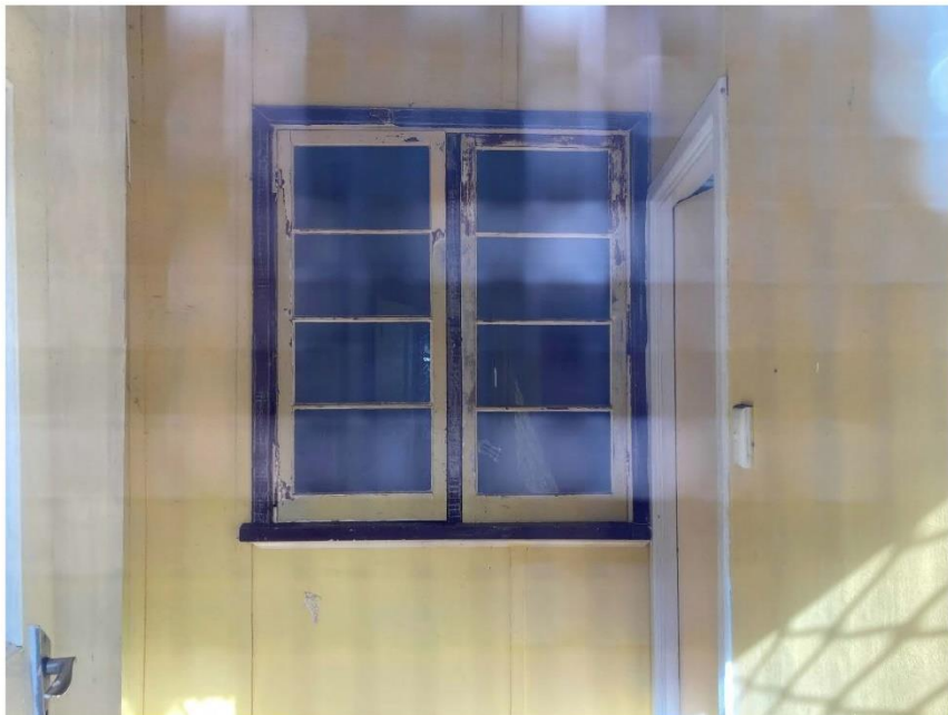
PHOTOGRAPH 6 Original timber window sill and asbestos clad timber framed wall visible where part of brick veneer wall has been removed
