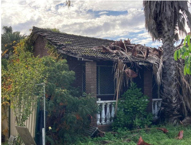
PHOTOGRAPH 1 Joslin Street elevation (south) showing deteriorated roof trims, eaves and bowing and collapsing section of roof.
