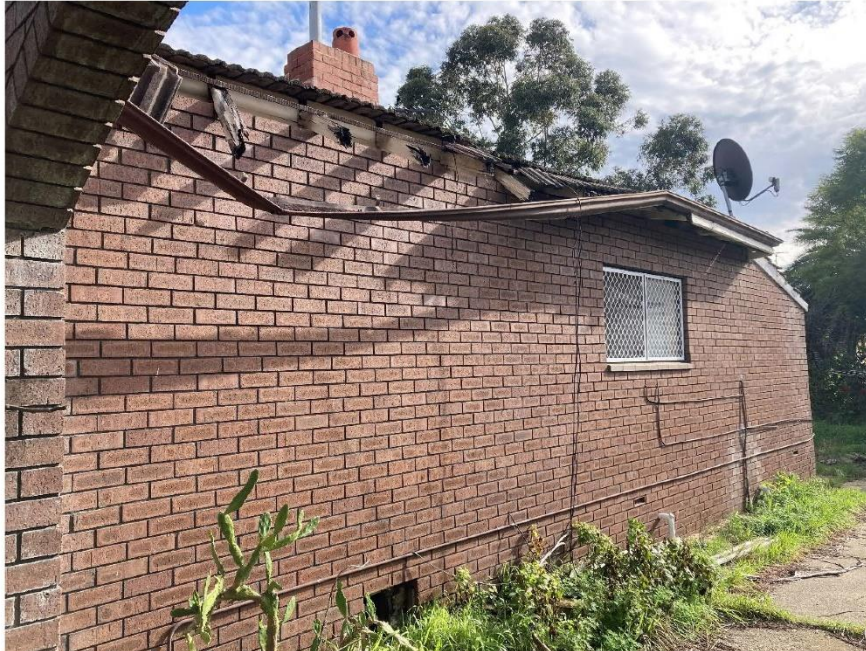
PHOTOGRAPH 4 – East elevation showing deteriorated gutter and collapsing eaves. Note sub-floor access hole to base of wall and the original red face brick chimney.
