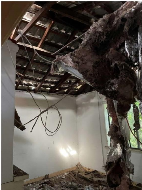
PHOTOGRAPH 10 Lounge showing collapse ceiling and bowing roof timbers. Light entering the roof space indicates a hole in the roof probably around the chimney.
