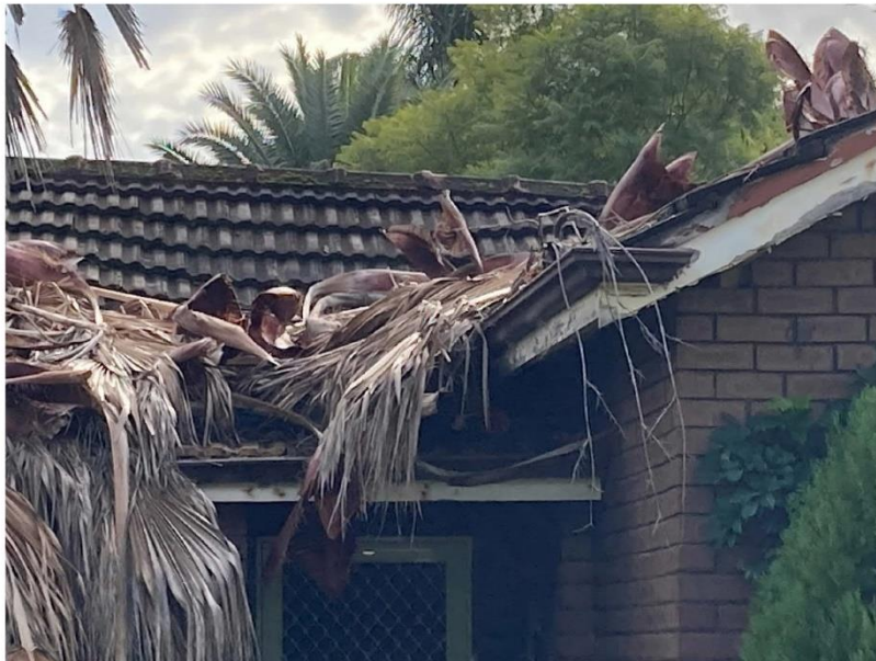
PHOTOGRAPH 2 Detail of collapsing section of roof above front entry hall
