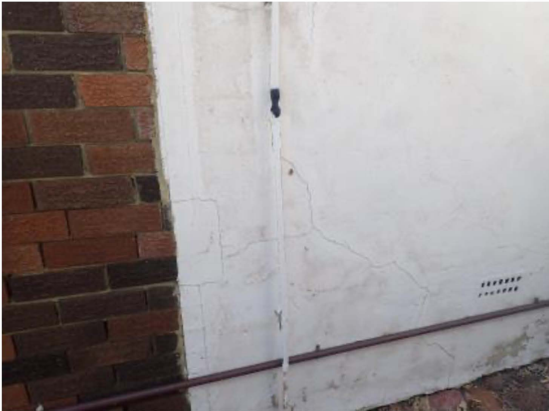
FIGURE 7 CRACK ADJACENT TO BRICK VENEER
