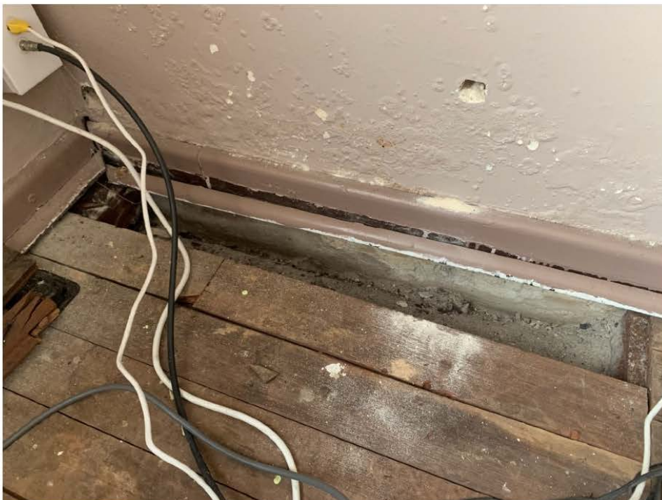
FIGURE 11 SKIRTING, FLOORBOARDS, DRUMMY PLASTER AND CONCRETE FOOTINGS
