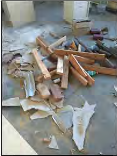
Plate 5: Broken FRP pieces lying on the ground within Building M.
