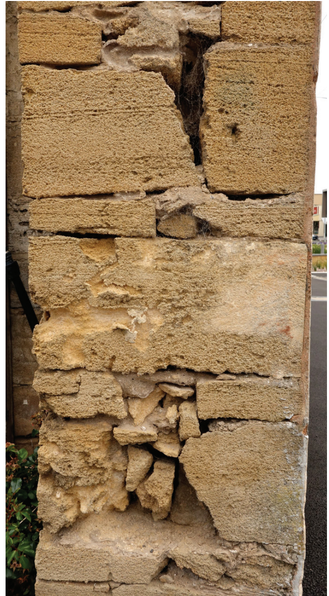
Sawn section through a solid wall of a similar limestone to Fremantle's. Note the large voids in the core of the wall. Occasional 'through stones' bond the outer and inner leaves together.
