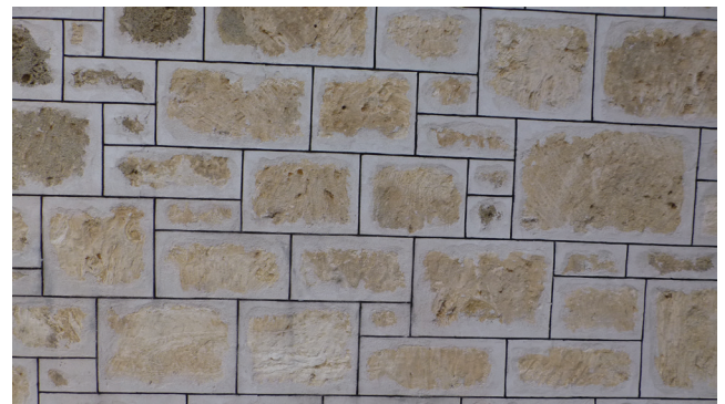
Squared random rubble with ruled joints; the incised lines were often painted (which was known as 'pencilling').
