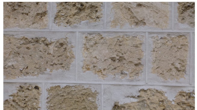
Ashlar blockwork with ribbon pointing; the raised ribbon is similar to tuck pointing of brickwork.
