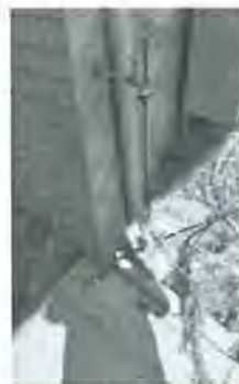
Downpipes draining against house walls- recommend soakwells
