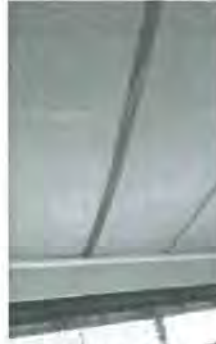
Large cracking to ceiling on porch
