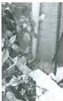
Downpipes draining against house walls- recommend soakwells
