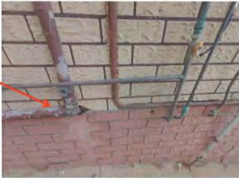
HEATING SYSTEM - NORTH WALL
