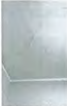
Large cracking to ceiling in kitchen area
