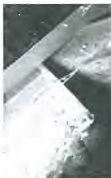
Old electric wiring system in roof space. Electrocution hazard.
