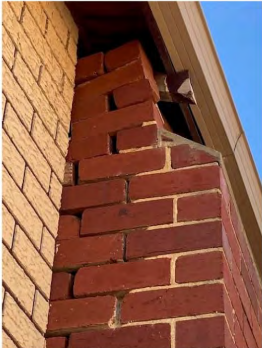
Brick chimney with deteriorated pointing, south wall.
