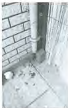
Downpipes draining against house walls- recommend soakwells
