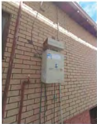
HEATING SYSTEM - NORTH WALL
