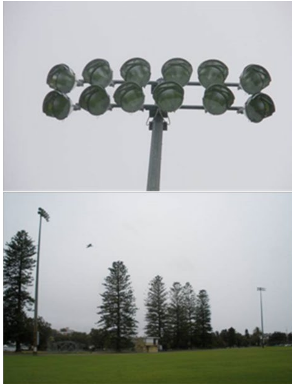
RIVER SIDE Musco floodlights on 30 m poles
