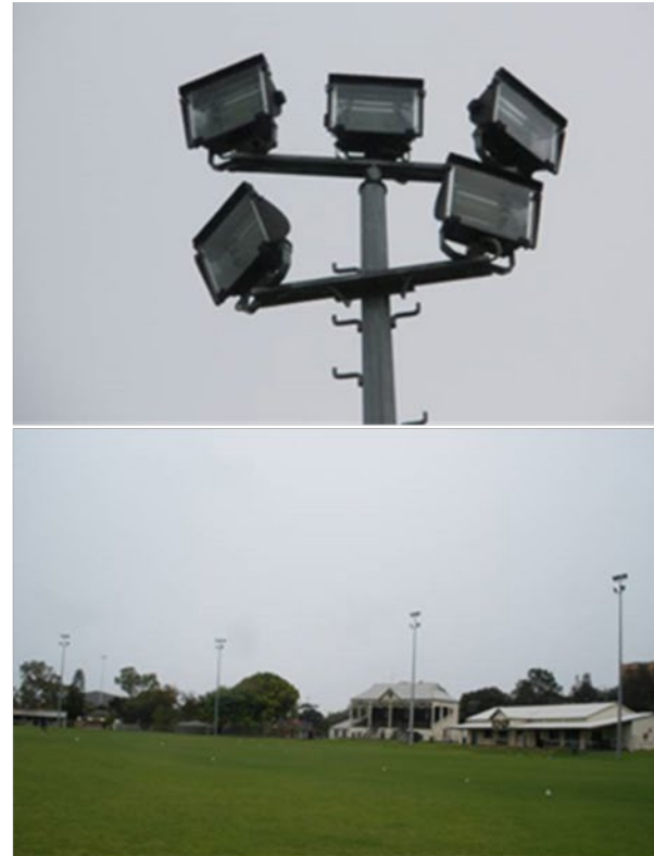
JOHN STREET SIDE Brightline floodlights on 20 m poles
