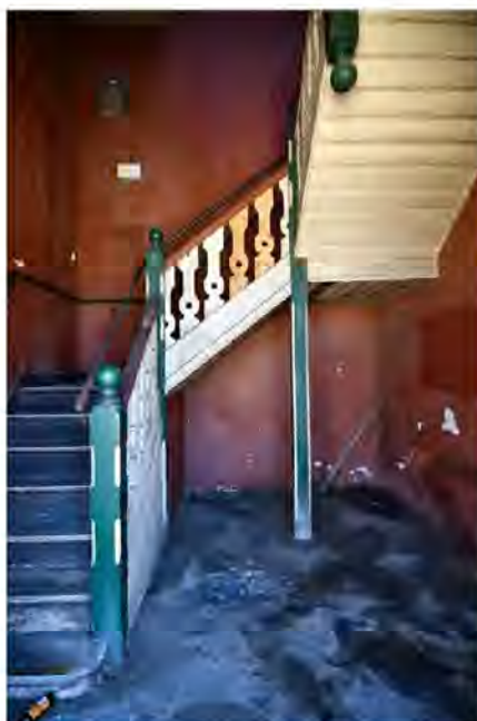
Photograph 35 Victoria Pavilion southern stairs. Griffiths Architects December 2021 . Though in disrepair the stairs are intact. The masonry is much affected by damp.
