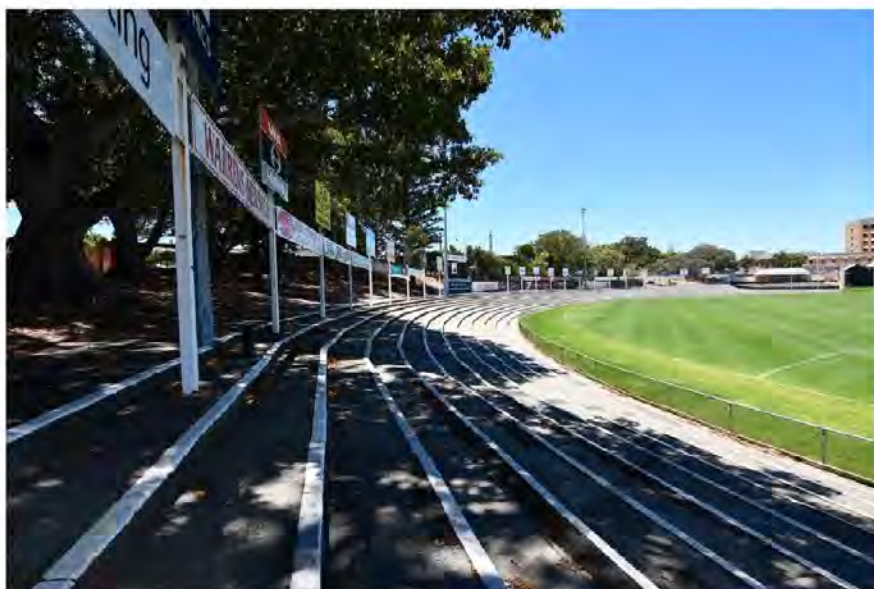
Photograph 30 Concrete terraces and advertising signs. Griffiths Architects December 2021 The terraces are formed by precast concrete kerbs and concrete paving slabs. These are in very poor condition and in some locations are badly displaced.
