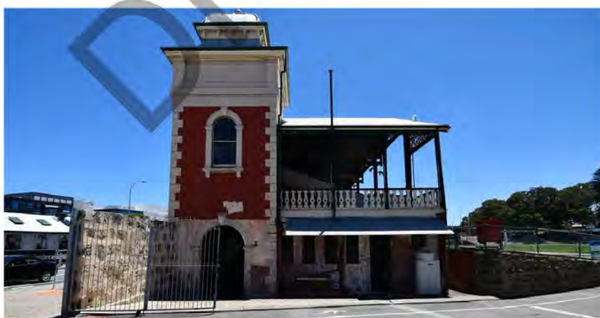
Photograph 32 Victoria Pavilion south elevation. Griffiths Architects December 2021. This embankment and limestone walls are later additions, increasing the pitch of the bank substantially.
