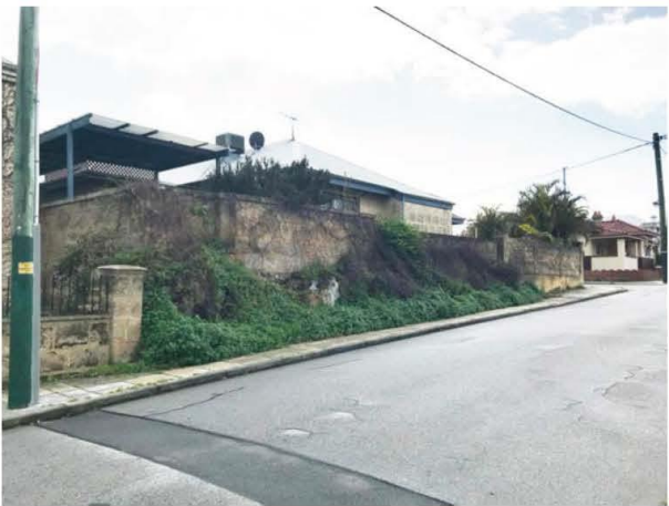
09. 21 TRAFFORD ST (SUBJECT SITE) - EXISTING HIGH LIMESTONE FENCE ON EXPOSED REMNANT LIMESTONE TO MARTHA ST. EXISTING OUTDOOR LIVING SPACE WITH NO SETBACK TO SOUTH WEST CORNER
