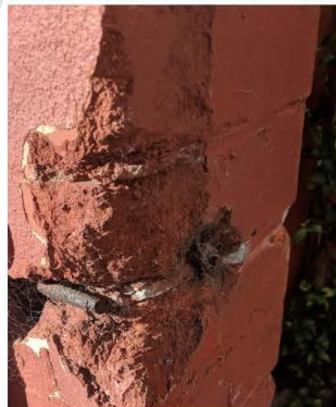
7.3.6 Example of damage to brickwork and deteriorating steel from acrylic paint trapping moisture and salts in the wall.
