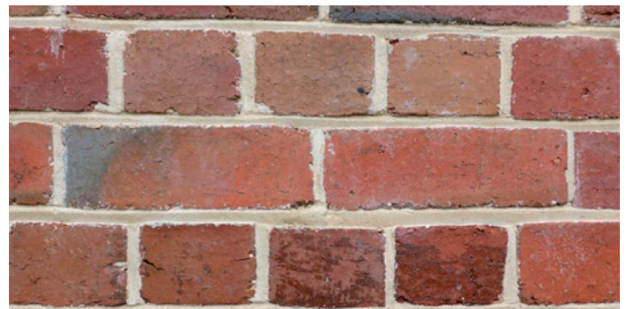
English bond - Alternating courses of header and stretcher bricks indicate solid wall construction.
