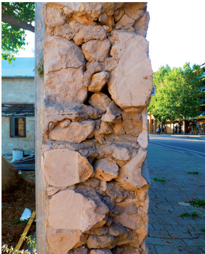
Cross section showing typical solid limestone wall construction. The outer leaves of larger squared stones are tied together with occasional through stones and the central core is loosely filled with small pieces of rubble and mortar — often leaving large voids.
