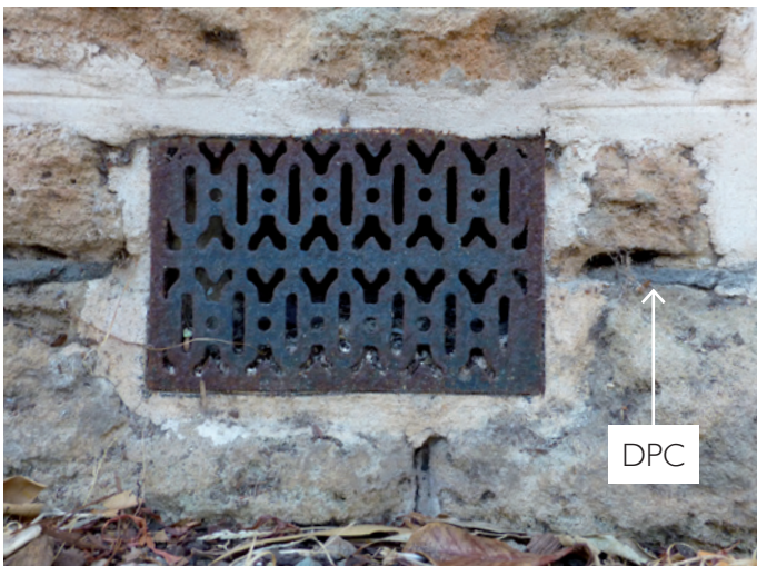
Traditional bituminous damp proof course and underfloor ventilation in solid limestone wall.
