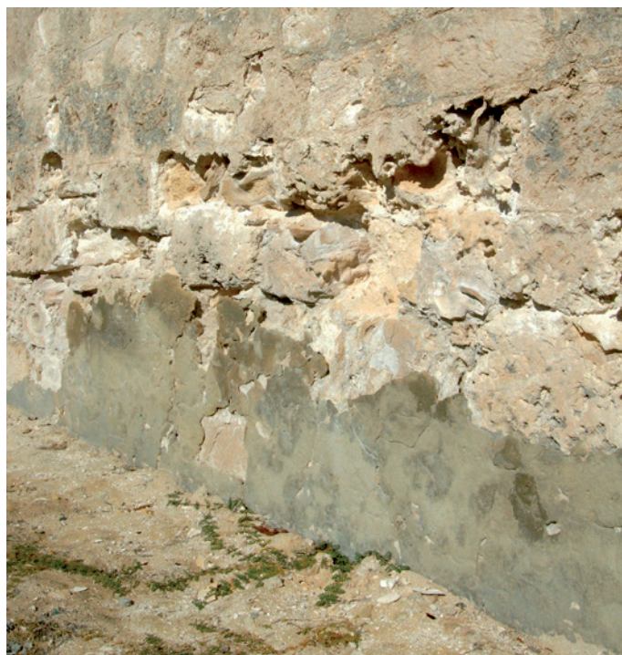
Salt attack — typical damage to the base of a limestone wall. Attempts to stop the decay by patching with cement has only driven the dampness further up the wall. (Photograph: David Young)
