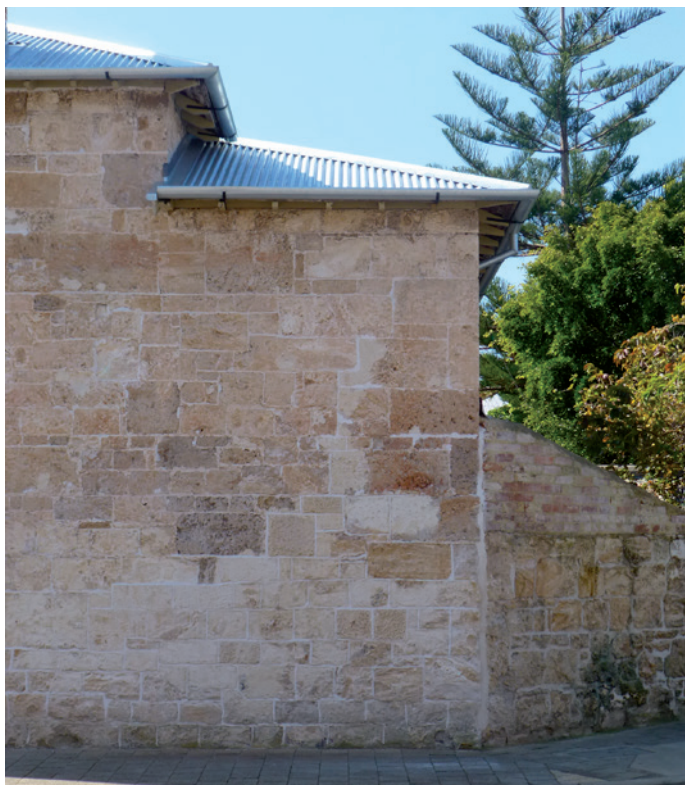
Solid stone wall after remedial works – refer to page 2 for the 'before' photo.
