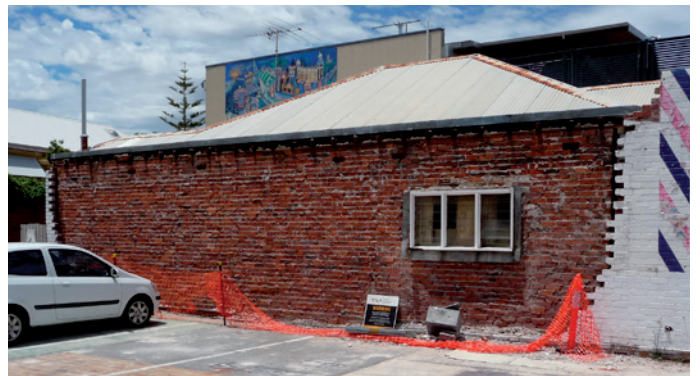
Cavity construction building where the outer leaf (painted white) collapsed because the cavity wall ties rusted away in the damp outer leaf of the wall leaving this leaf unbraced and unstable. The paint was part of the problem — had there been no paint the outer leaf would not have been so damp.
