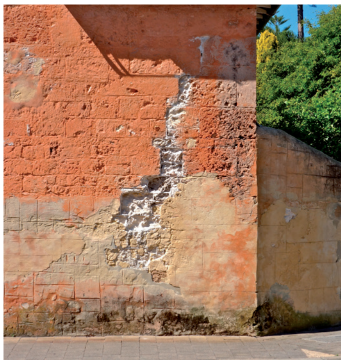
Falling Damp - Severe decay of limestone due to a corroded gutter directing water down the wall face.
