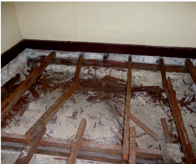
Collapsed, rotten timber floor where external wall vents were blocked by the later addition of a concrete verandah floor.
