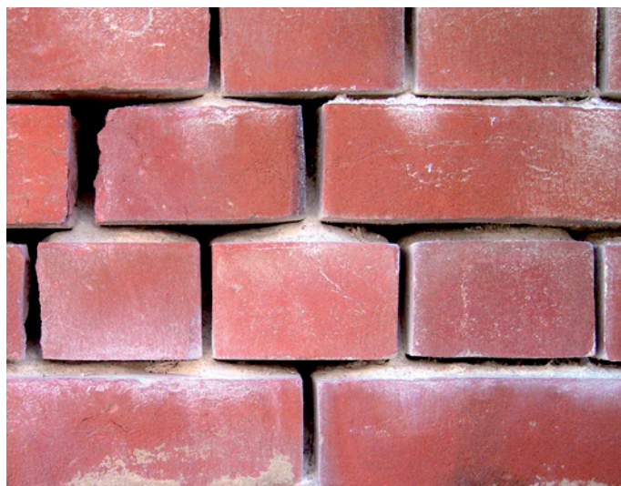
This wall has a severe case of rising damp and salt attack and needs urgent attention. While it may seem that there is a problem with the mortar, in fact the permeable lime mortar has protected the bricks by acting sacrificially. The correct approach to repair is to repoint the joints in a lime mortar. (Photograph: David Young)
