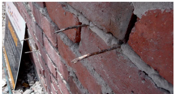
Rusted steel wall ties from the example above.
