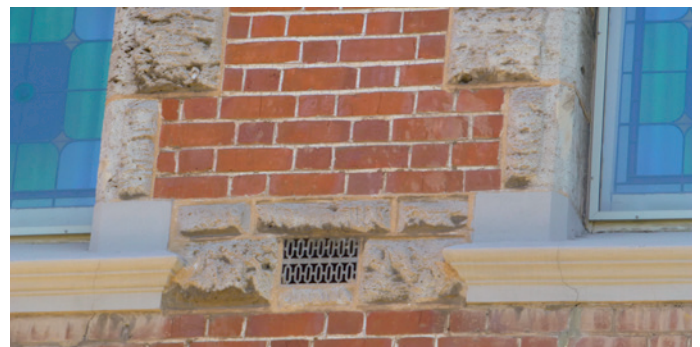
Flemish bond - Alternating header and stretcher bricks in each course generally indicate solid wall construction.
